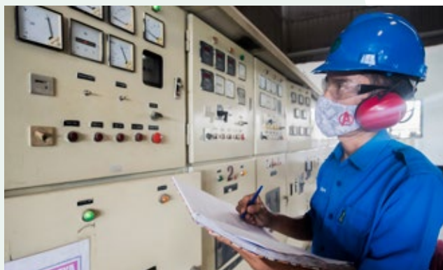
Energy usage monitoring in Belani Elok Mill, South Sumatra
